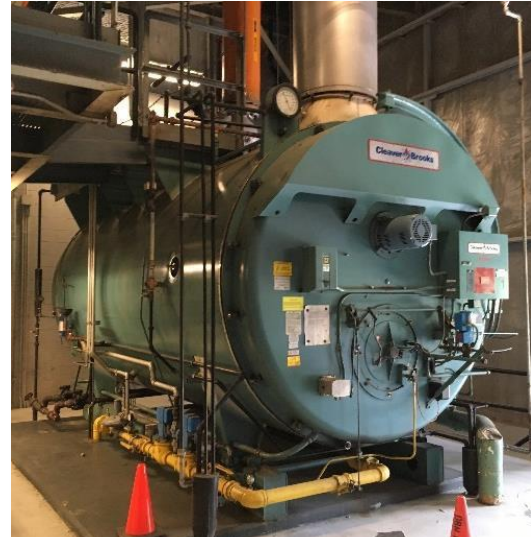
Eliminating the two existing massive steam boilers that operated at only 70% efficiency compared to 95% efficient new boiler technology.
