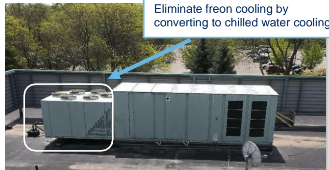
Old rooftop HVAC unit with old inefficient air-cooled air conditioning replaced with high-efficiency water-cooled systems
