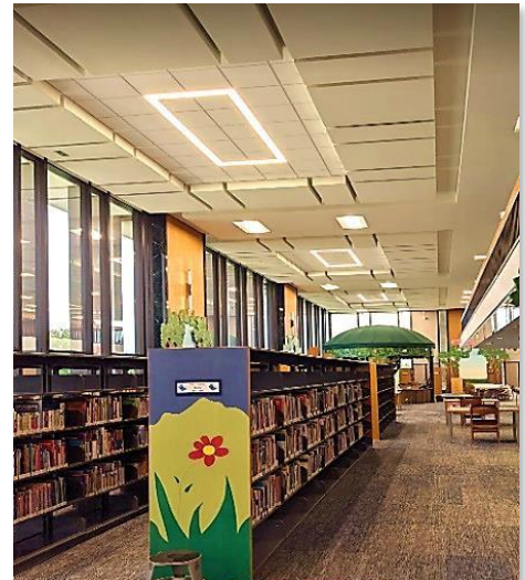
New library LED lighting
